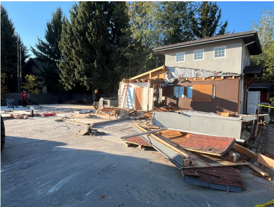
Figure 2 Site condition observed upon issuance of the stop work order.
