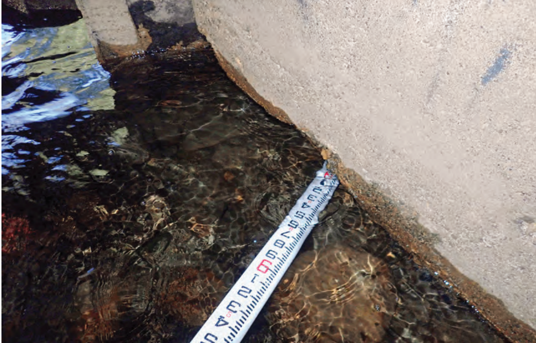
Undermining at northeast corner looking northeast.
