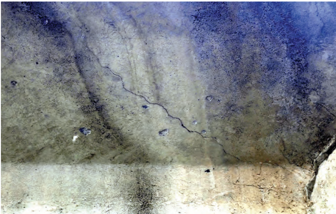
Cracks in flanges at east abutment.
