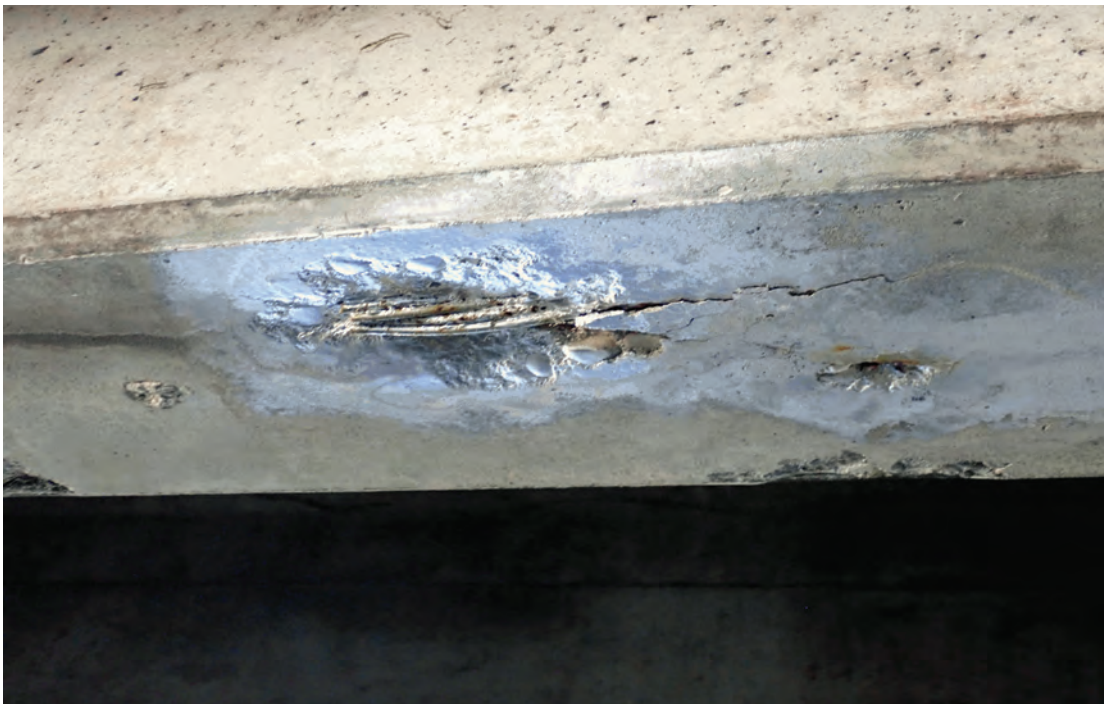
Exposed prestressing looking north.
