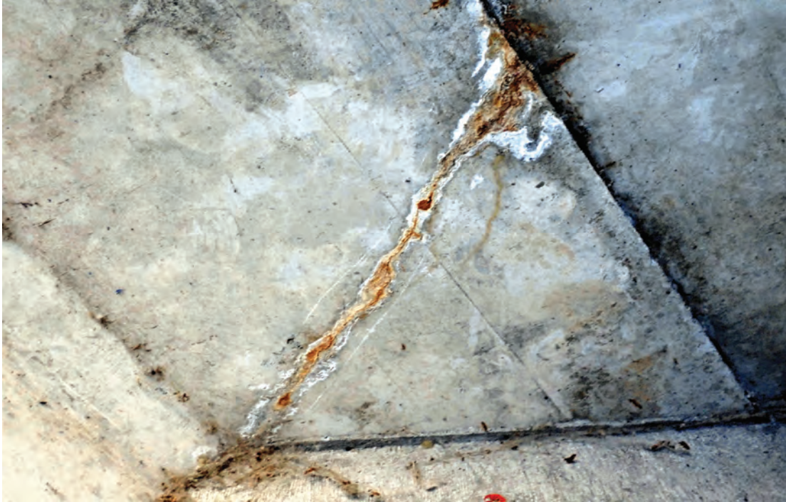
Cracks in flanges at east abutment.
