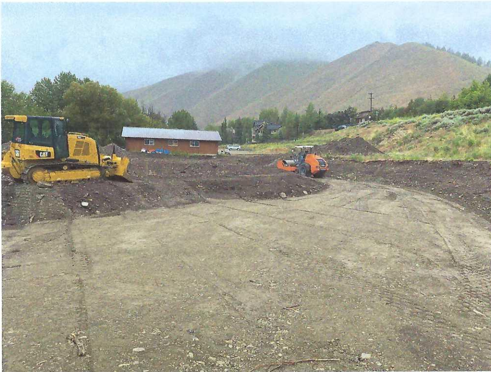
Imported sand and gravel placed in 10" loose lifts, watered and compacted with multiple passes of a vibrating smooth drum roller as structural fill. 29Jun20
