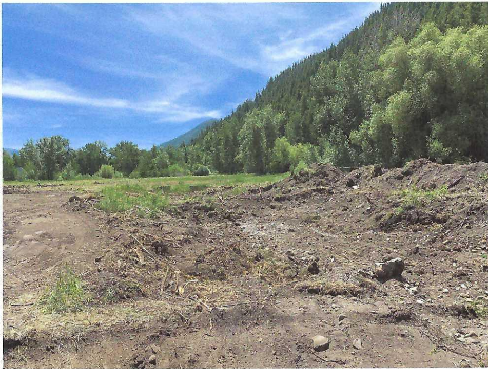
Organics, debris and disturbed soils to be removed prior to placing structural fill to match adjacent existing grade. 26Jun20
