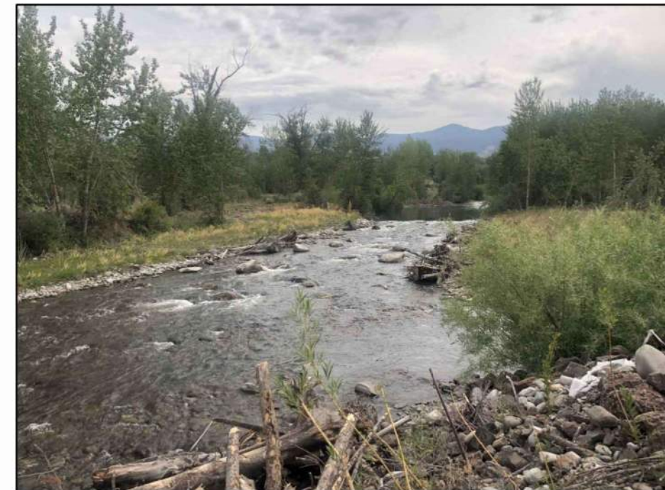
CONSTRUCTED RIFFLE ON THE LEMHI RIVER WITH BANK TREATMENTS - ONE YEAR AFTER CONSTRUCTION.
