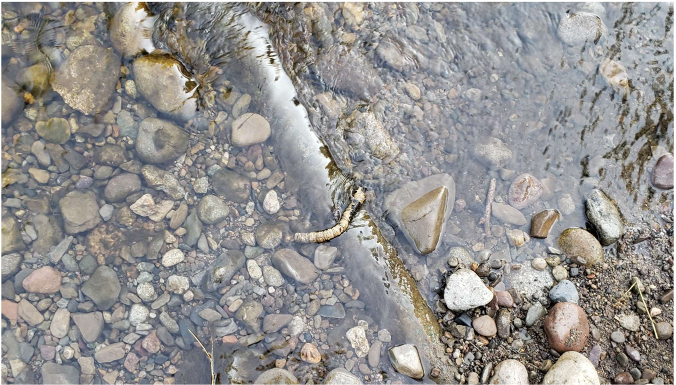
Figure 3-4. Pipe exposed in the creek bed adjacent to the existing irrigation diversion.
