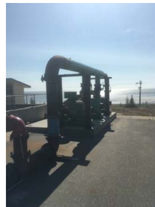
Temp Blowers moved out and running
