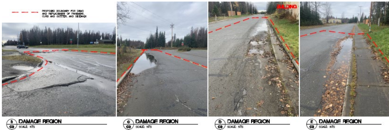
First Street typical damaged areas
