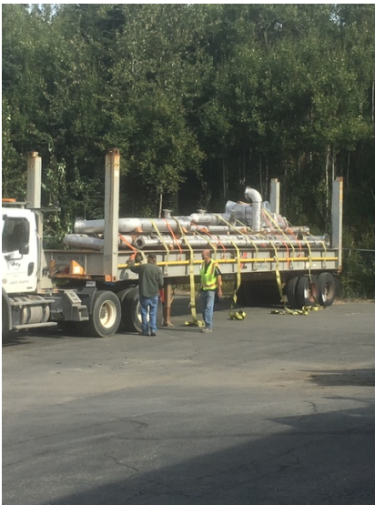
Stainless Piping on Site
