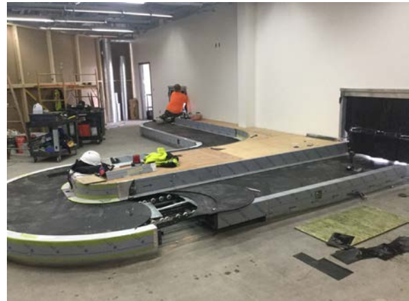
New Baggage Conveyor
