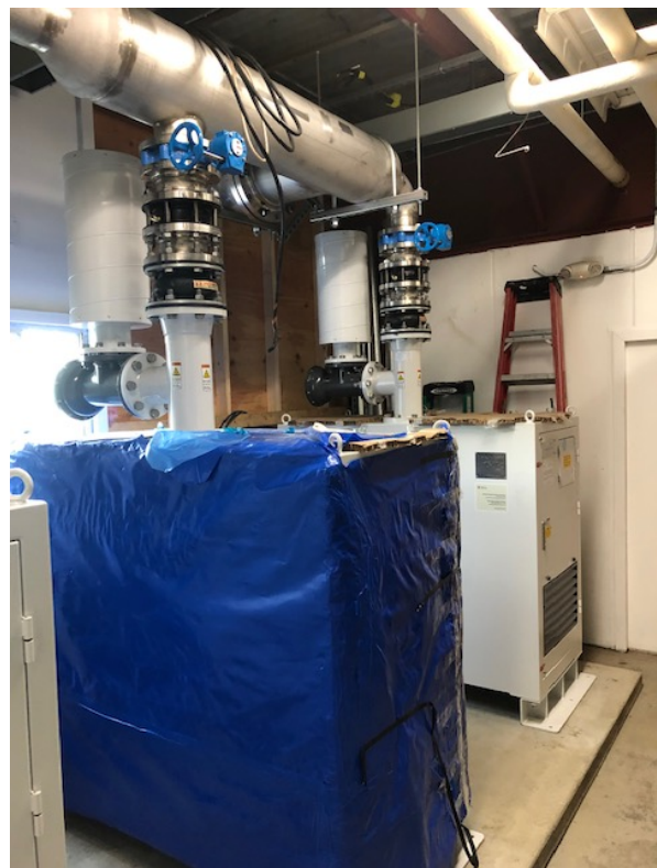
New Blowers installed
