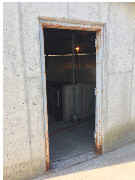
Old Doors Rusted through
