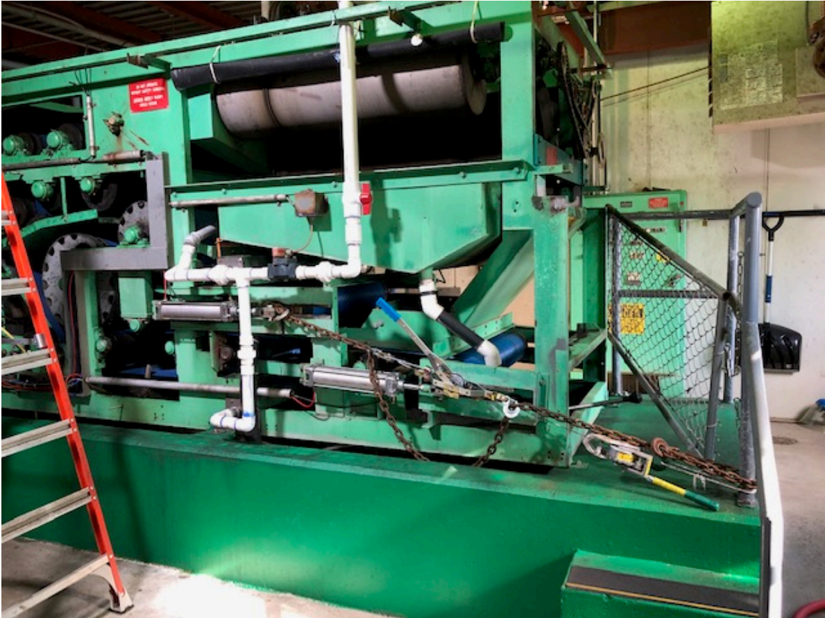
Existing Sludge Belt Press
