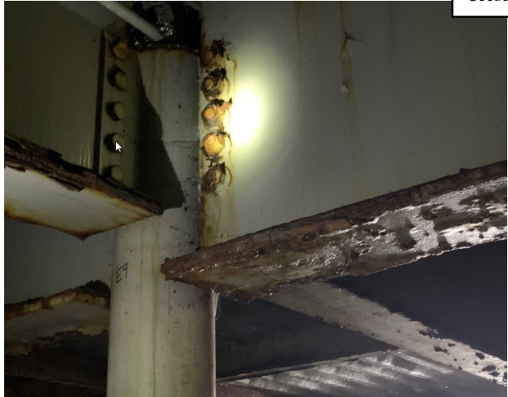
10. Corrosion at connecting bolts. This is the central 9" diameter support column for the roof between the two effluent tanks.
