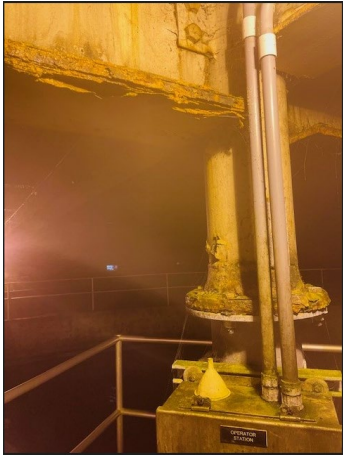
3. Corrosion of the steel beam and connection at the clarifier basin.
