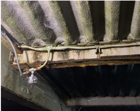
7. Underside view of metal roof decking. Foam insulation is saturated with water. Note Algae growth.
