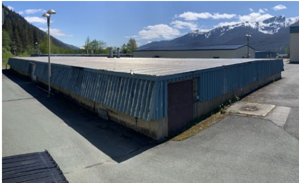
8. Low slope metal roof missing fasteners, lacks water drainage via gutters and downspouts.
