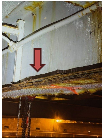
2. Corrosion at primary structural I-beam. Note significant corrosion at bottom flange causing delamination of the steel.
