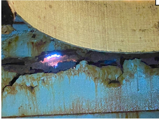
4. Corrosion of metal framing at the roof vent exhaust opening. Note daylight showing.
