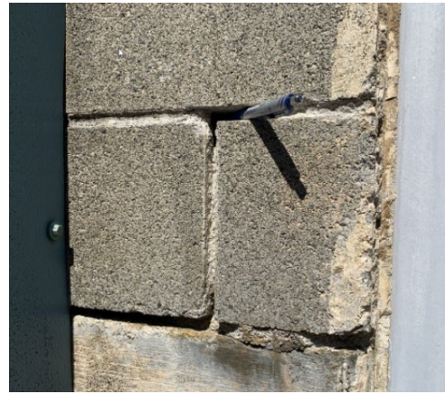
6. Mortar at concrete blocks has deteriorated. Spalling due to winter freeze-thaw cycles evident.
