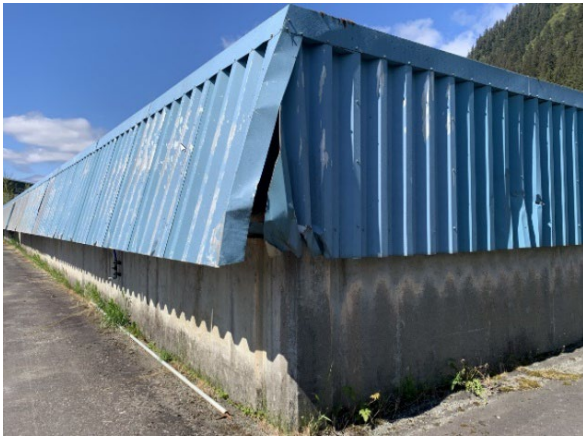
5. Numerous holes and gashes in 1973 metal siding are open to the interior of the building.
