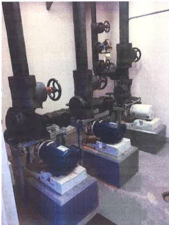
Mountainside Estates Pump Station
