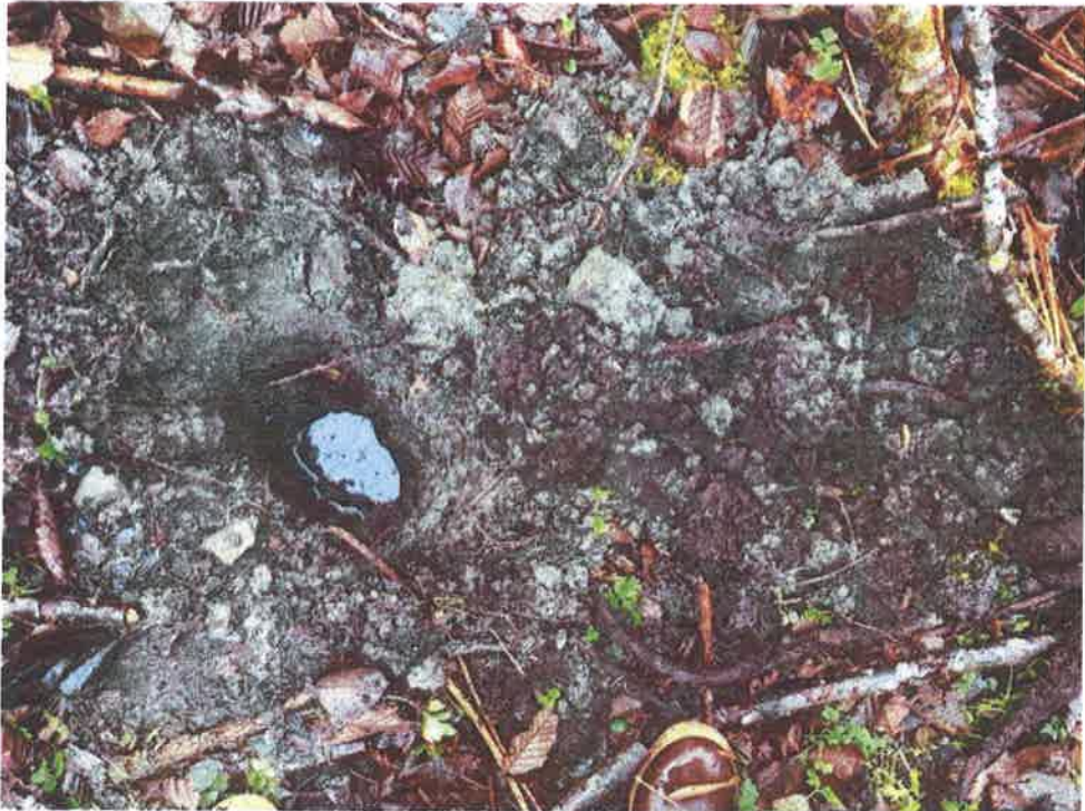
Photo 5 - Eroded fill material with silts and gravels over native organic soils at the toe of the fill pad.
