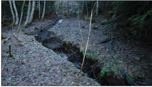
Figure 2.—Channel at toe of fill.
