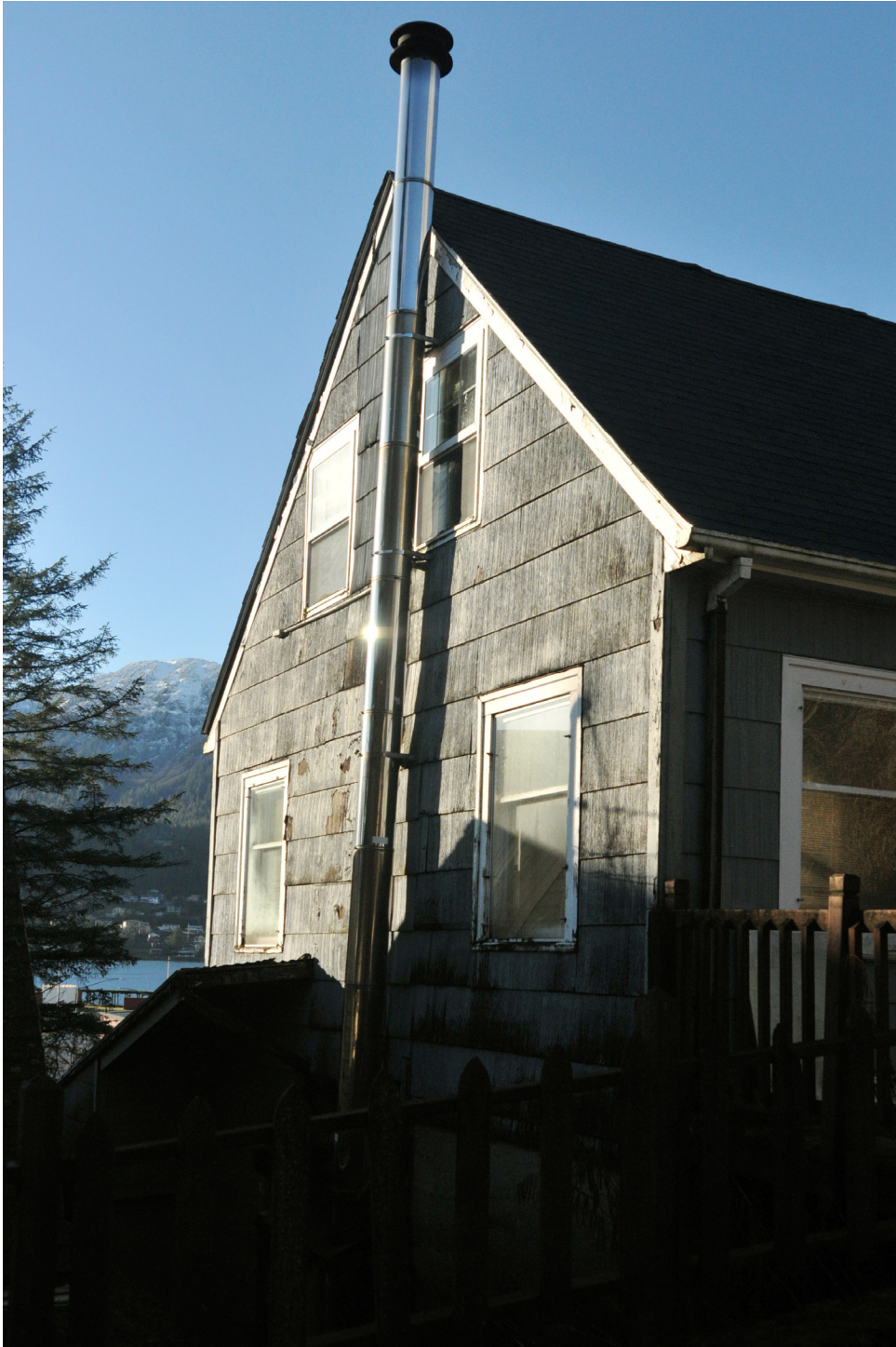
South Facade. A metal chimney has since replaced the original cement block chimney. Martin-Johnston House, 2023
