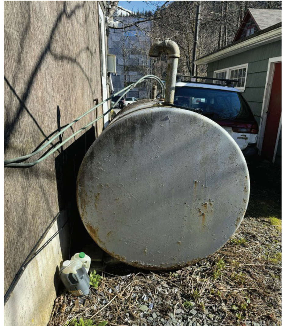
Fig. 20: Storage Tank at 203 West Third St.
