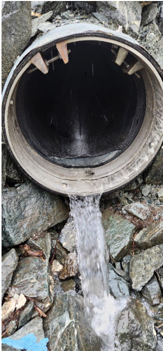
Figure 4 Image of the installed and functioning check valve – Meander at Northland Outfall
