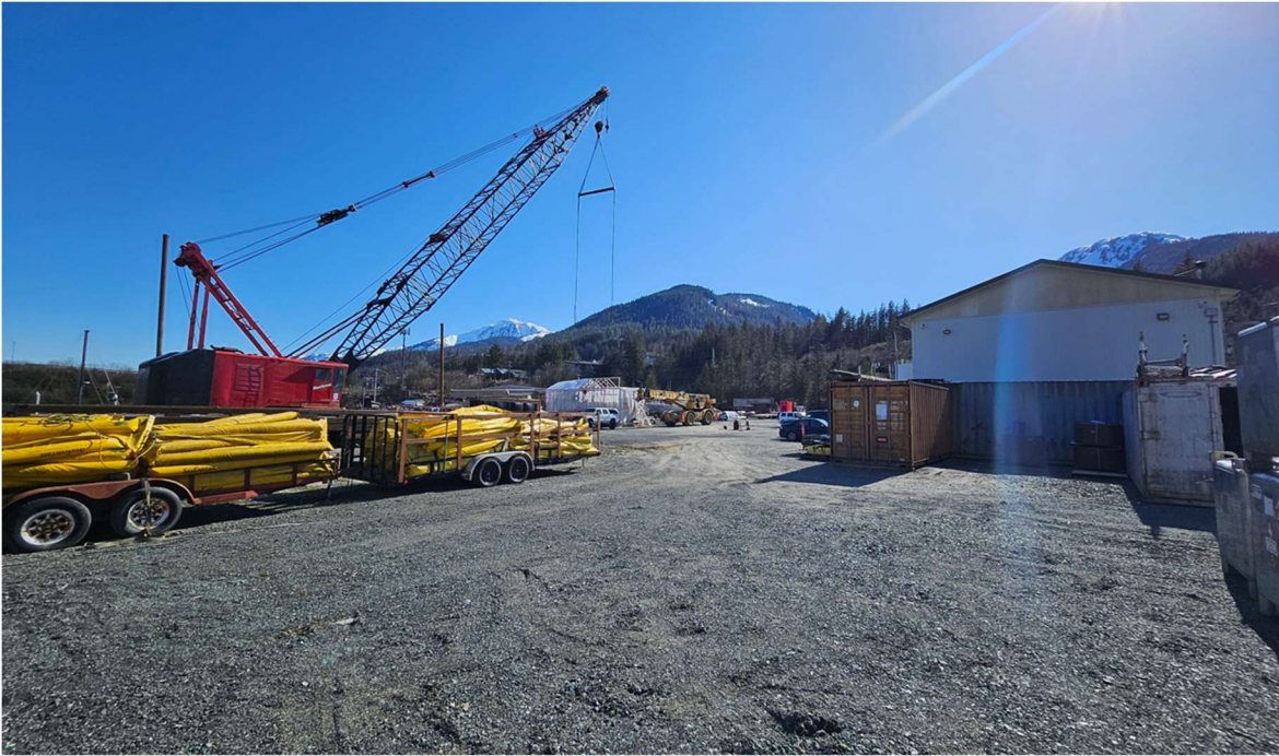
ADL 51488 looking SW down center of ATS 842 in its developed condition toward Douglas Island. (20240416_152631)
