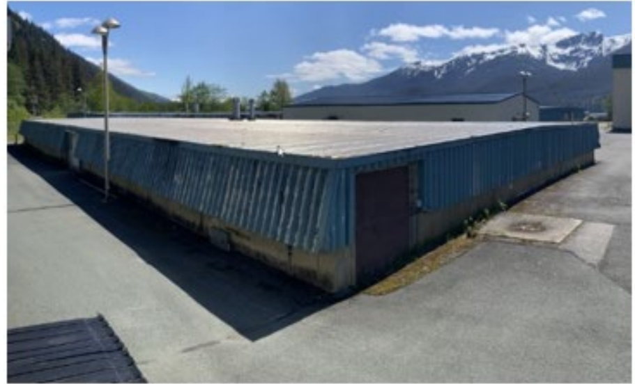
8. Low slope metal roof missing fasteners, lacks water drainage via gutters and downspouts.
