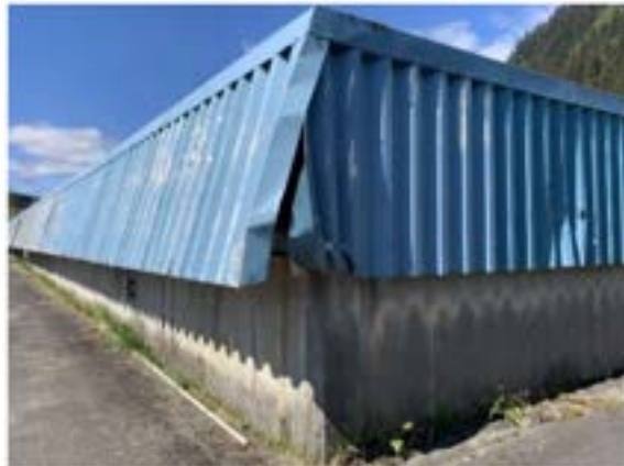
5. Numerous holes and gashes in 1973 metal siding are open to the interior of the building.
