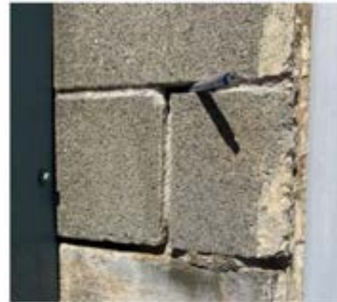
6. Mortar at concrete blocks has deteriorated. Spalling due to winter freeze-thaw cycles evident.
