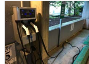
Marine Parking Garage EV Charging Station
