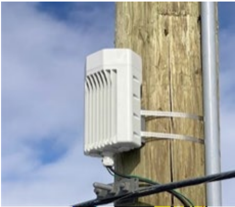
2 Example of a Wi-Fi access point mounted on a telephone pole.
