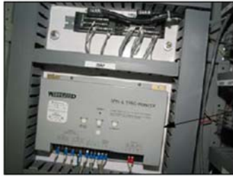
MASTER CONTROL CABINET
