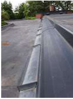
CR hail damage 2023 dents in copper edging.jpg 69K
