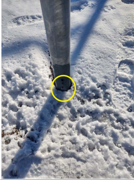
Ice Bridge Post #1 Ground Missing
