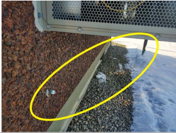
HVAC Ground Missing Before
