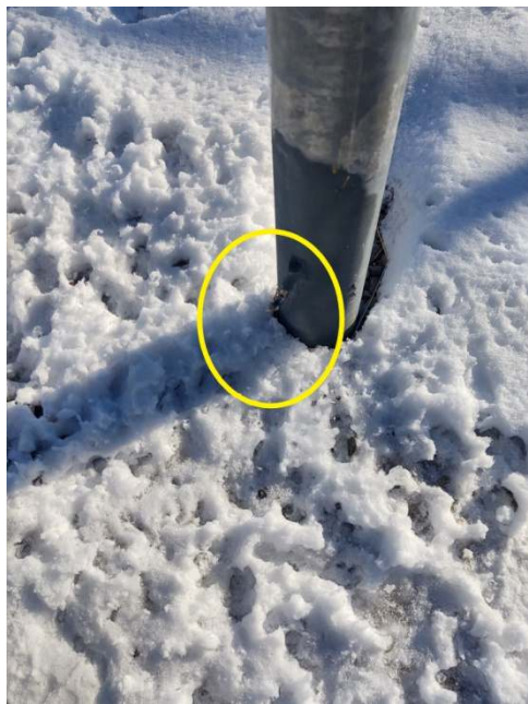
Ice Bridge Post #2 Ground Missing
