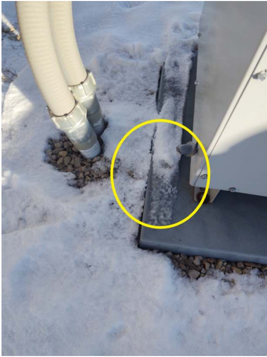
Isolation Transformer Ground Missing
