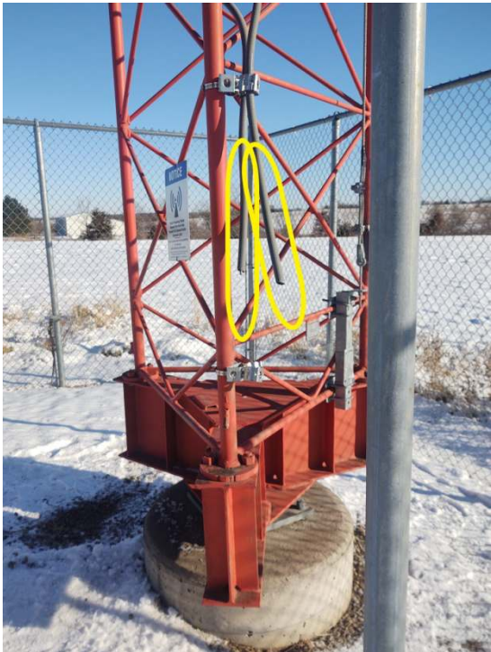
Tower Ground Bar Grounding Cables Missing
