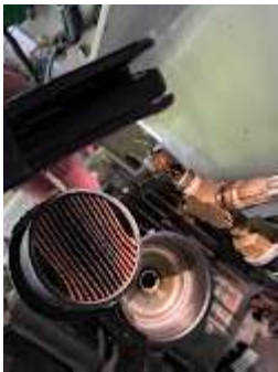
oil residue in filter and on blow off valve.JPG 2408K
