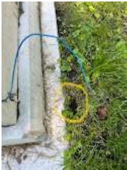
Where copper rod was.jpg 1716K
