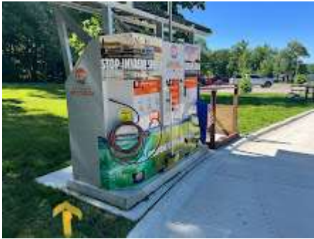
Arrow where copper ground rod.jpg 1165K
