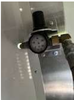
PSi gauge broken.JPG 2116K
