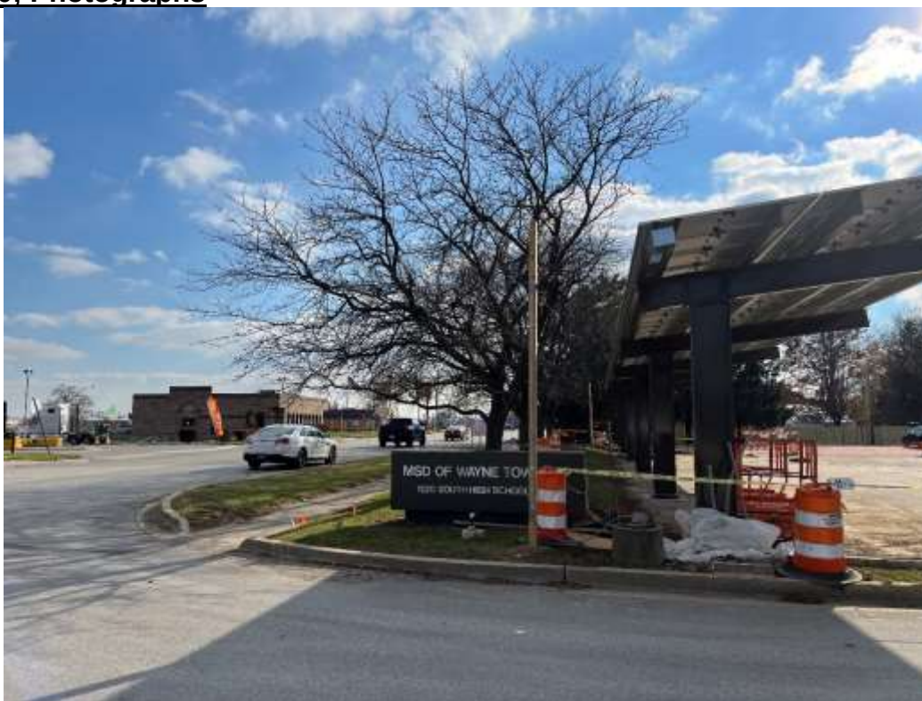
Photo looking south on subject site, at solar on carport in front yard.
