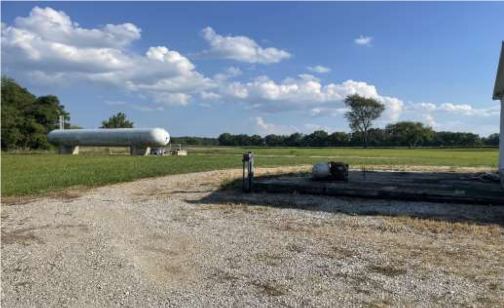
Photo Eight: Large Propane Storage Tank, Abutting Properties, Facing South
