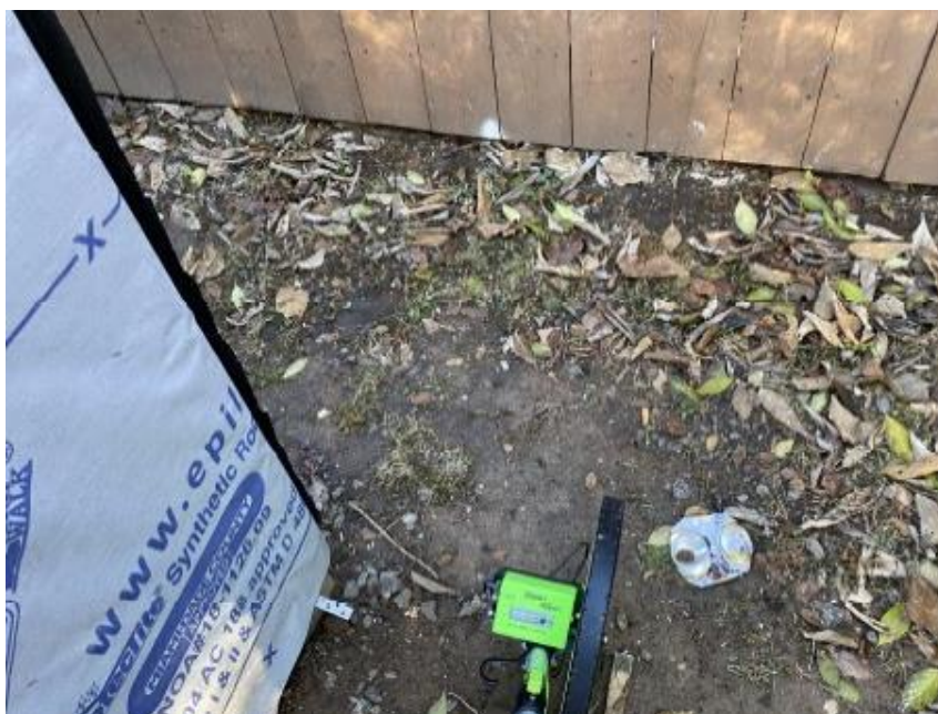
Photo 8: Separation Between Unpermitted Garage and Fence to East (November 2025)
