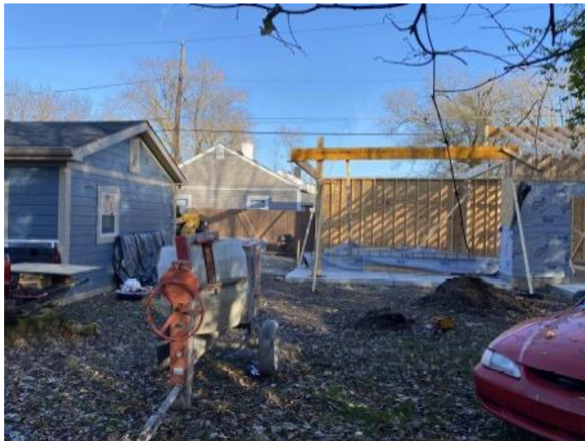
Photo 7: Unpermitted Garage Viewed from East (November 2025)
