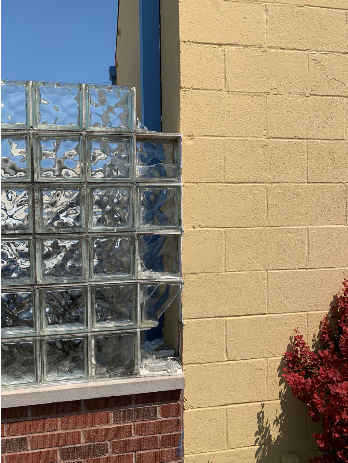
Photo of a section of the former fence showing disrepair – photo taken in May 2023
