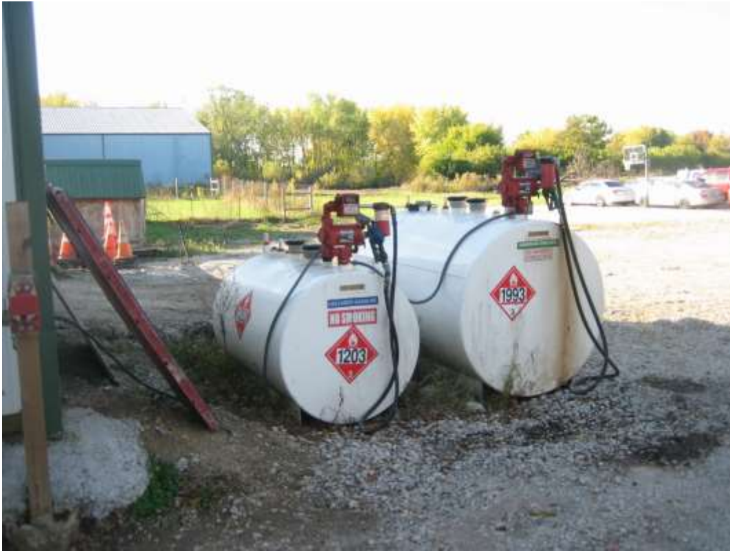
On-site fuel storage tank to the rear of existing barn, looking west.
