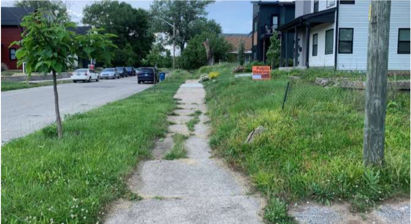
Condition of the sidewalk along the street frontage.
