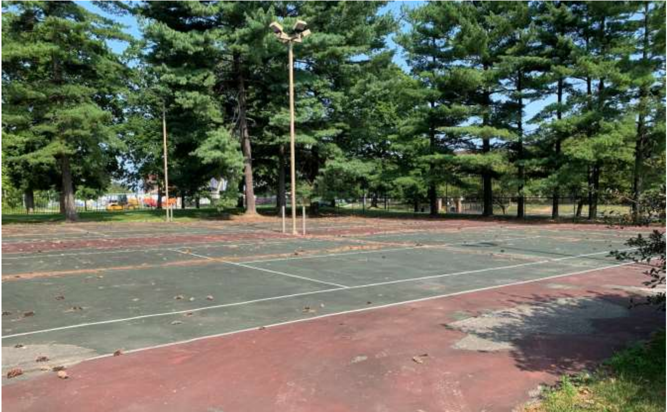
Close-up of the condition of the existing tennis courts to be removed.
