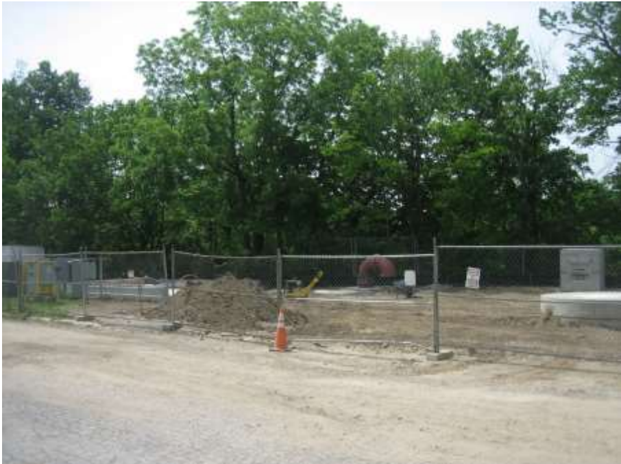
Photo of adjacent Fall Creek and 30 th Street Park under construction for combined sewer project, looking west.
