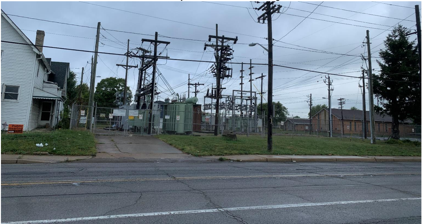
Photo of the electrical substation north of the site.
