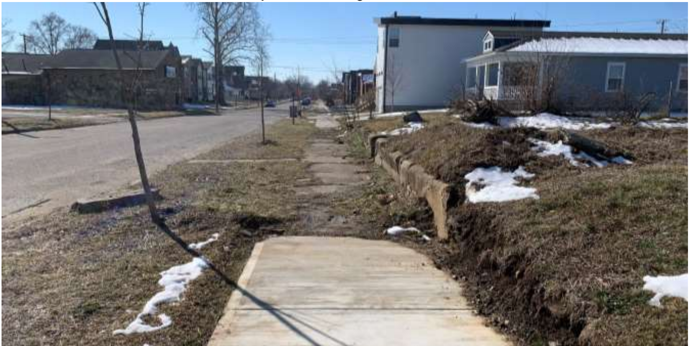
Photo of the sidewalk that would need to be repaired.
