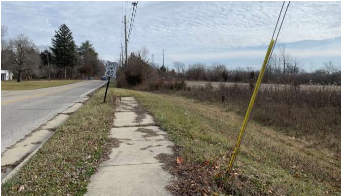
Photo looking east where the sidewalk ends along 46th Street.
