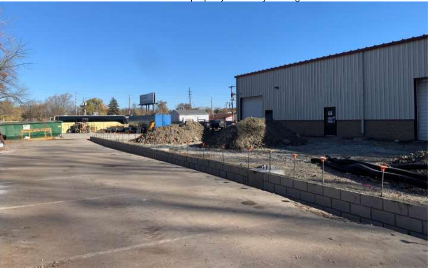
Photo of the existing west building façade and proposed building addition looking north.
