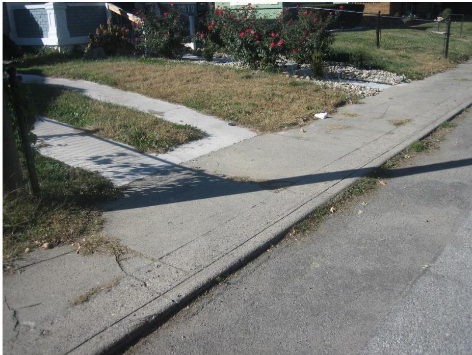
Photo 2 - Subject property existing low rise curb, that is driven over to access the non-permitted driveway, looking northwest.
