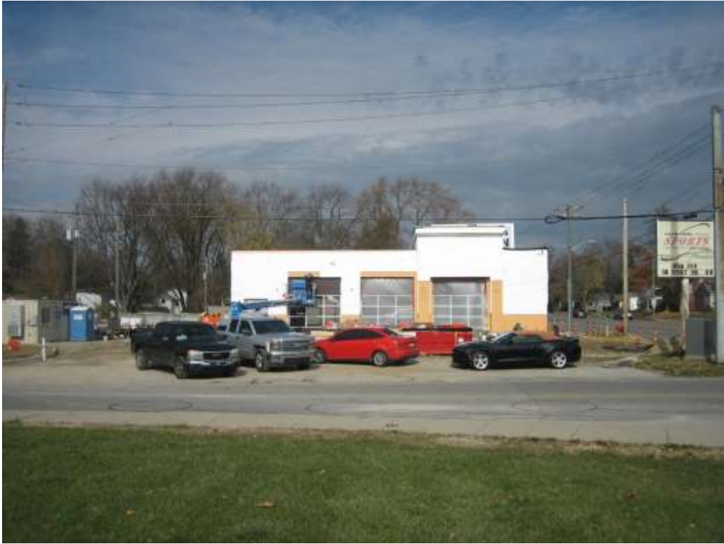
View of subject site, proposed building under construction, looking north from East 56 th Street.
