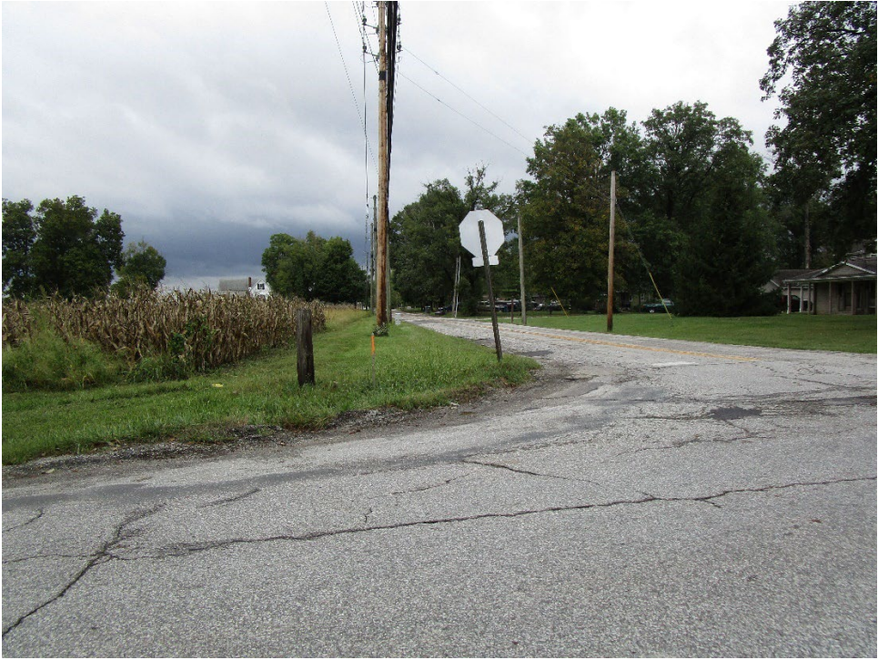
View looking north across intersection of East Southport Road and Hickory Road
