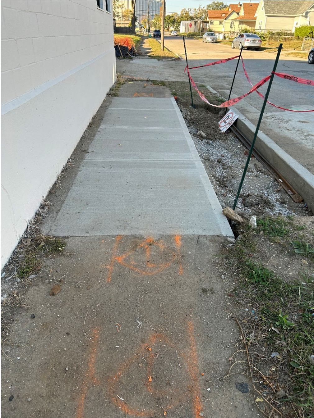
Photograph of sidewalk and subject alley (Part A), along Rembrandt Street, looking north
