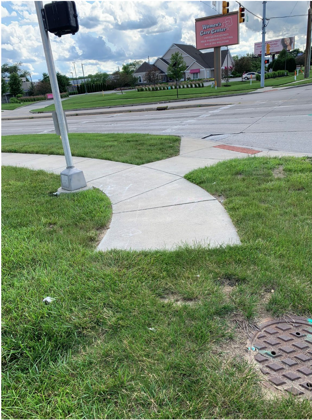
Existing sidewalk at 86 th Street and Georgetown Road intersection– sidewalk begins at this location and runs south
