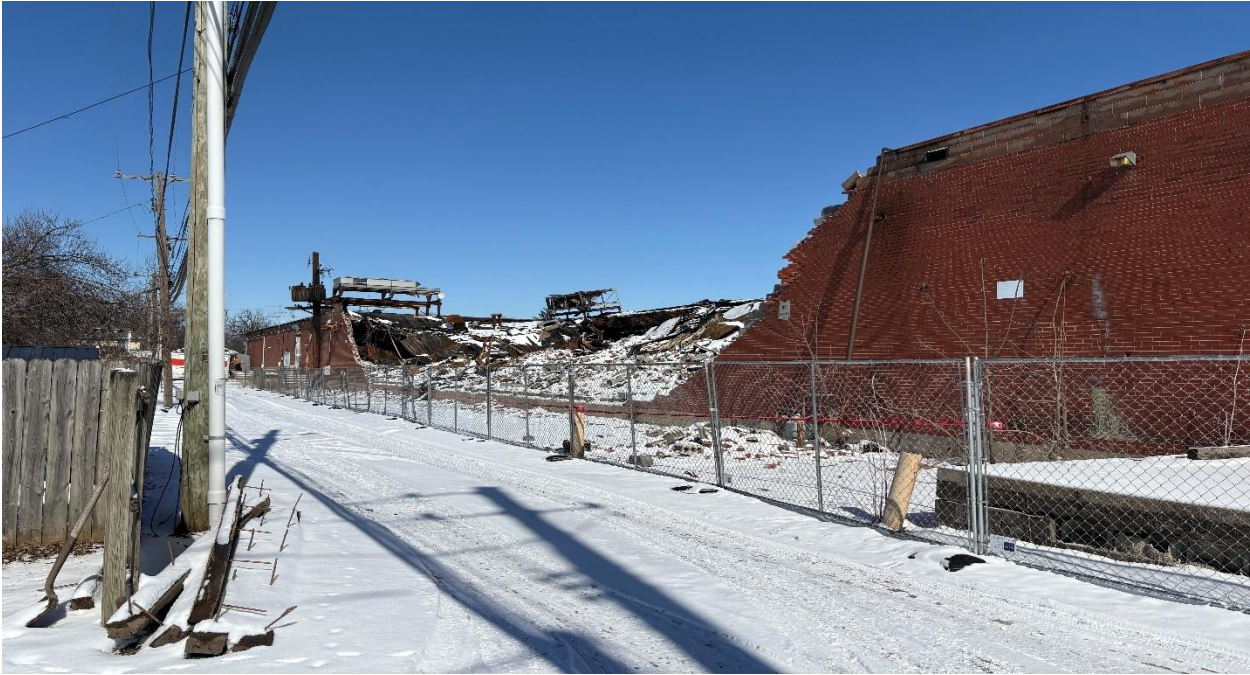
Photo Nine: Rear of Former Marsh Supermarket, After Fire Damage
