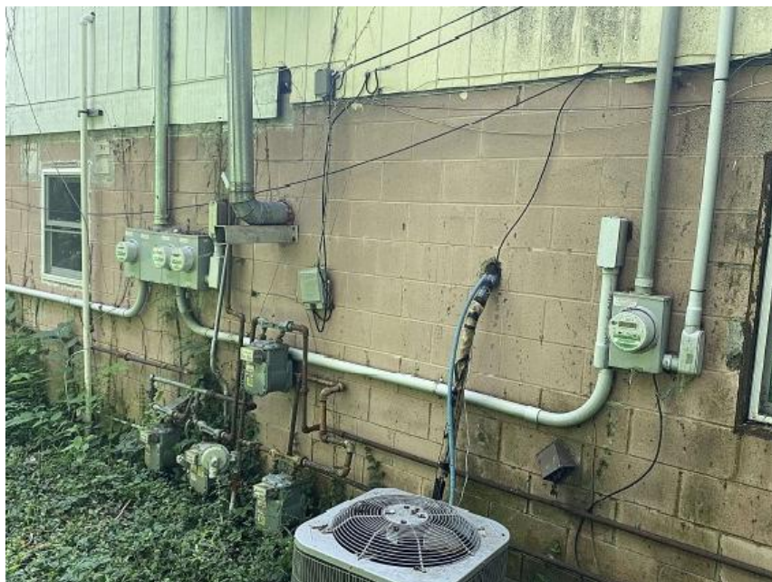
Photo 6: Multiple Power Meters on Multi-Family Building
