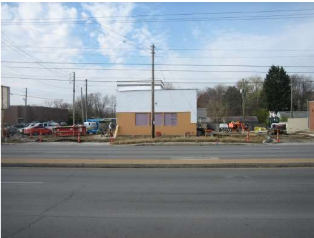
View of subject site, proposed building under construction, looking west from North Keystone Avenue.
