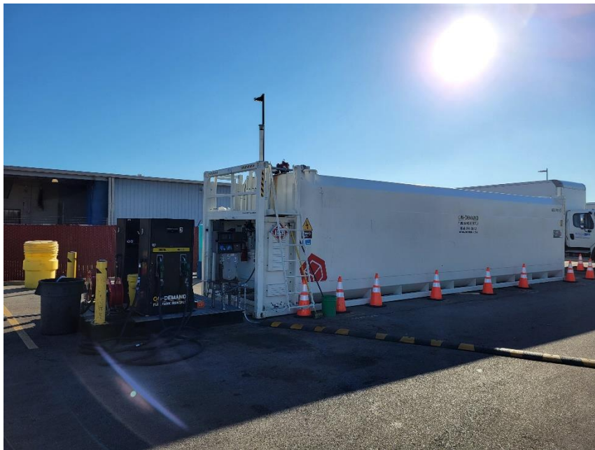
Photo 6: Temporary Fueling Station at Northeast of Property
