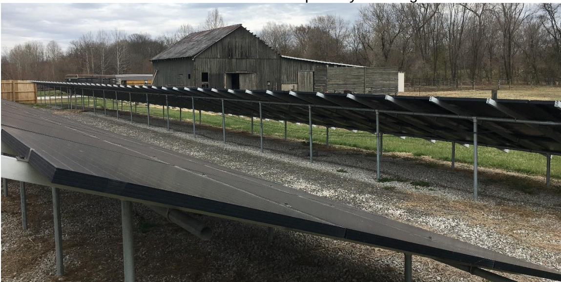
Solar panels on side/rear yard, looking east
