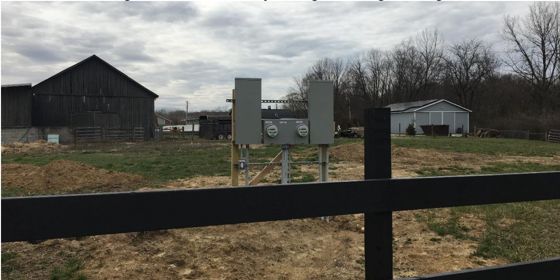
Utility meter, looking west
