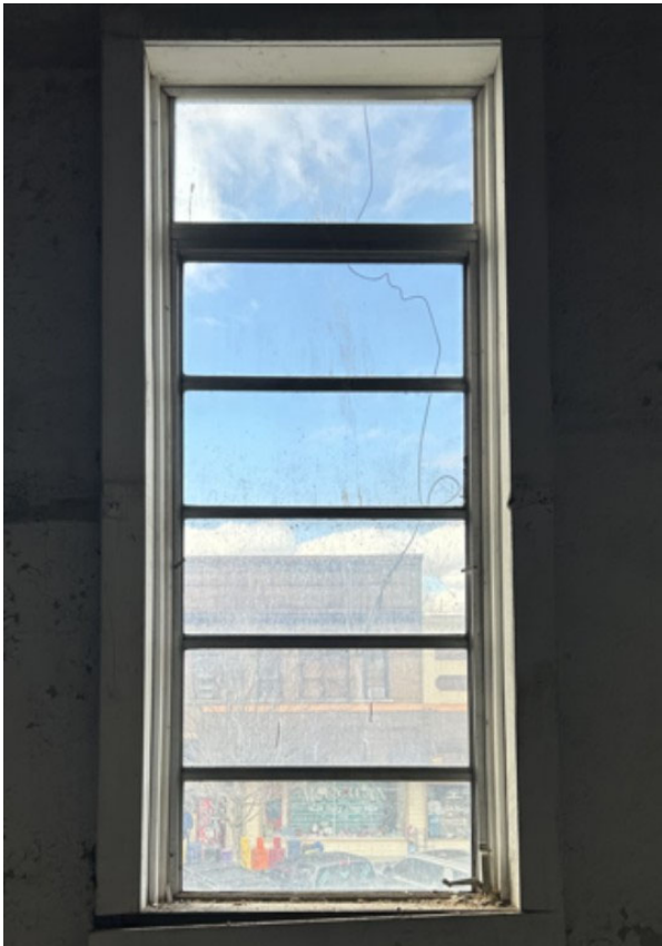
Applicant provided imagery of damaged windows
