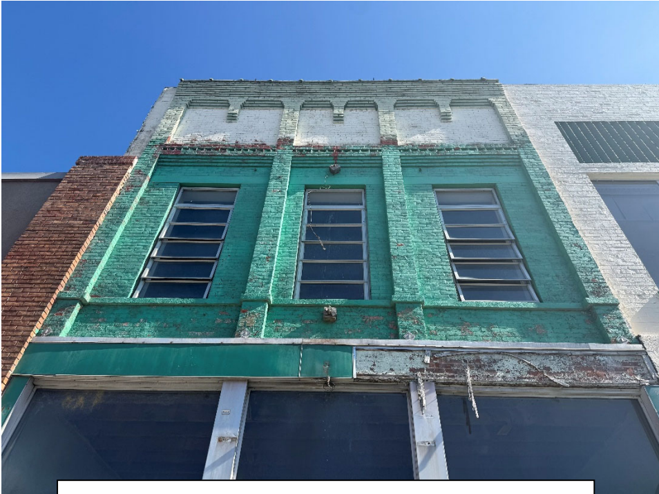
Upper façade detail showing damage
