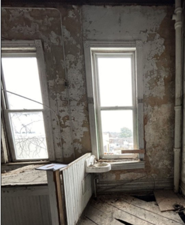
Applicant provided imagery of damaged windows
