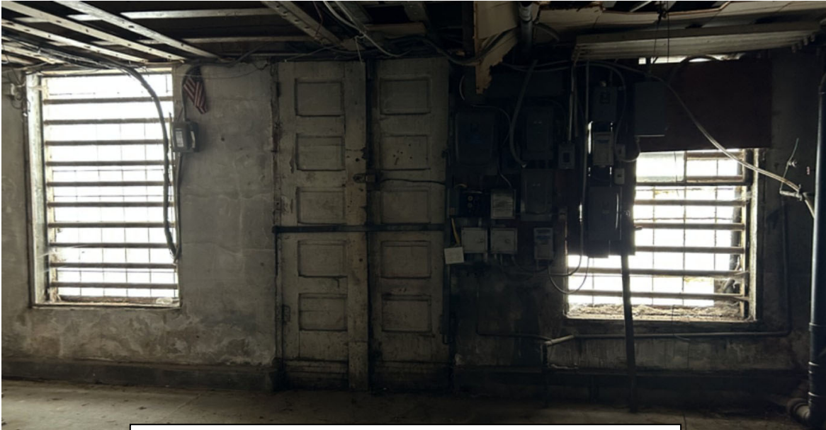
Applicant provided imagery of damaged windows
