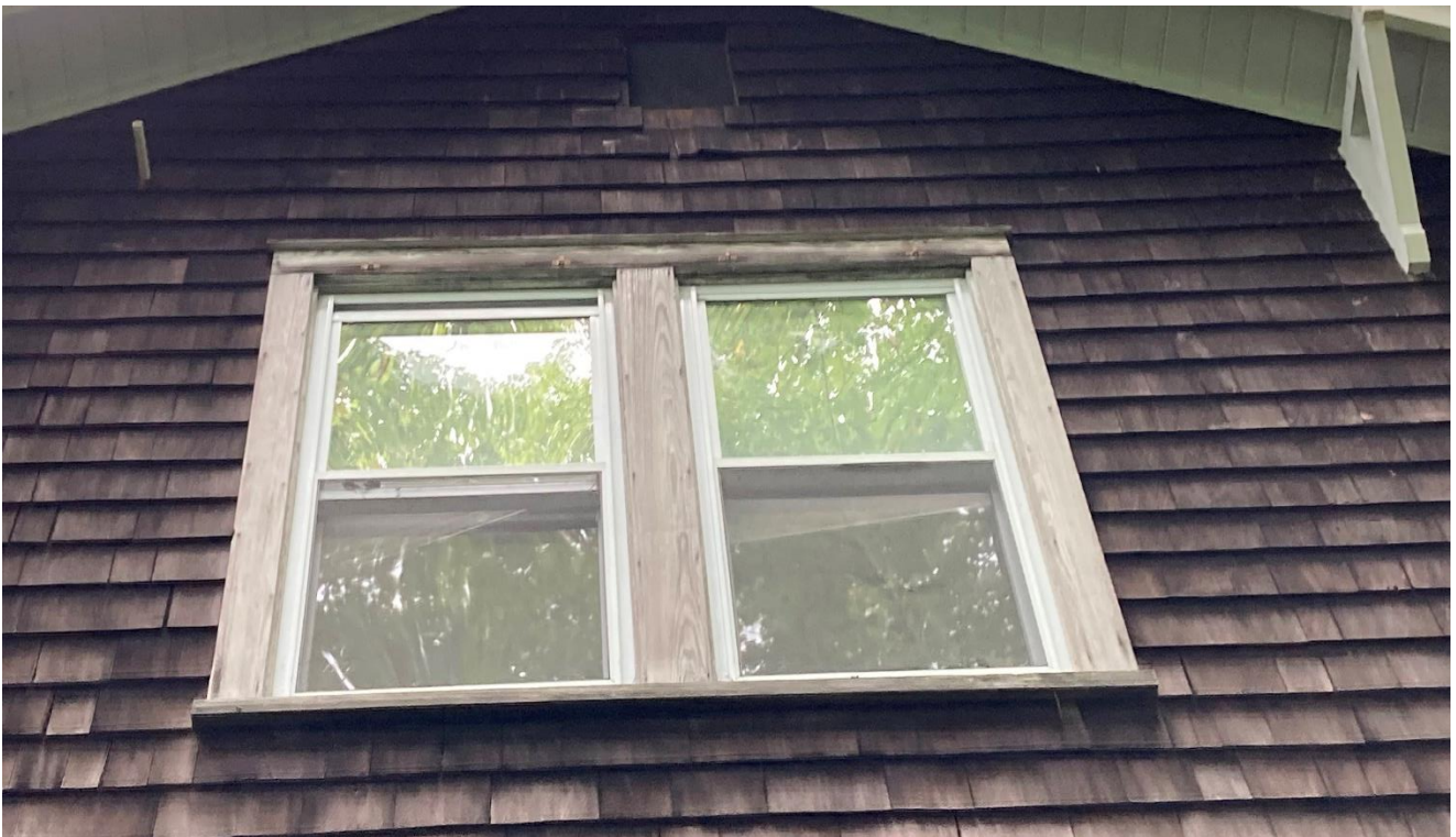
Figure 10 - Exposed/Unpainted Wood Window Trim
