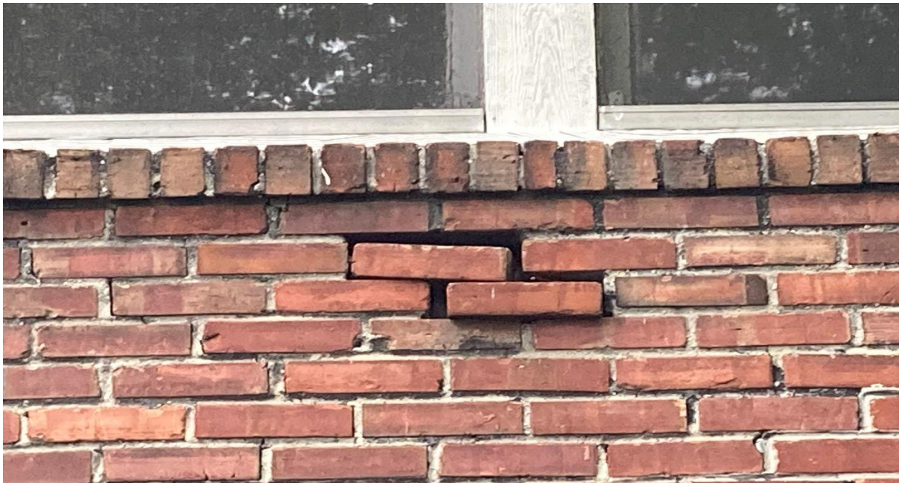
Figure 4 - Missing Mortar/Loose Brick
