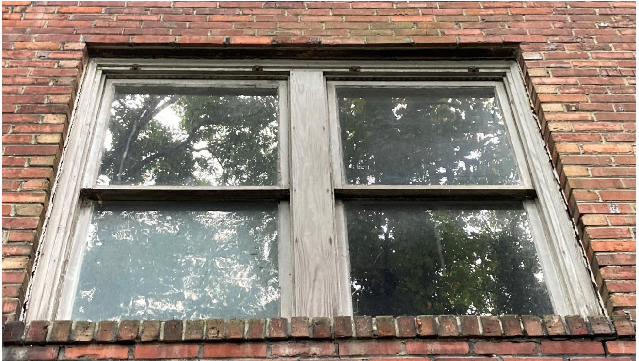
Figure 9 - Exposed/Unpainted Wood Window Trim
