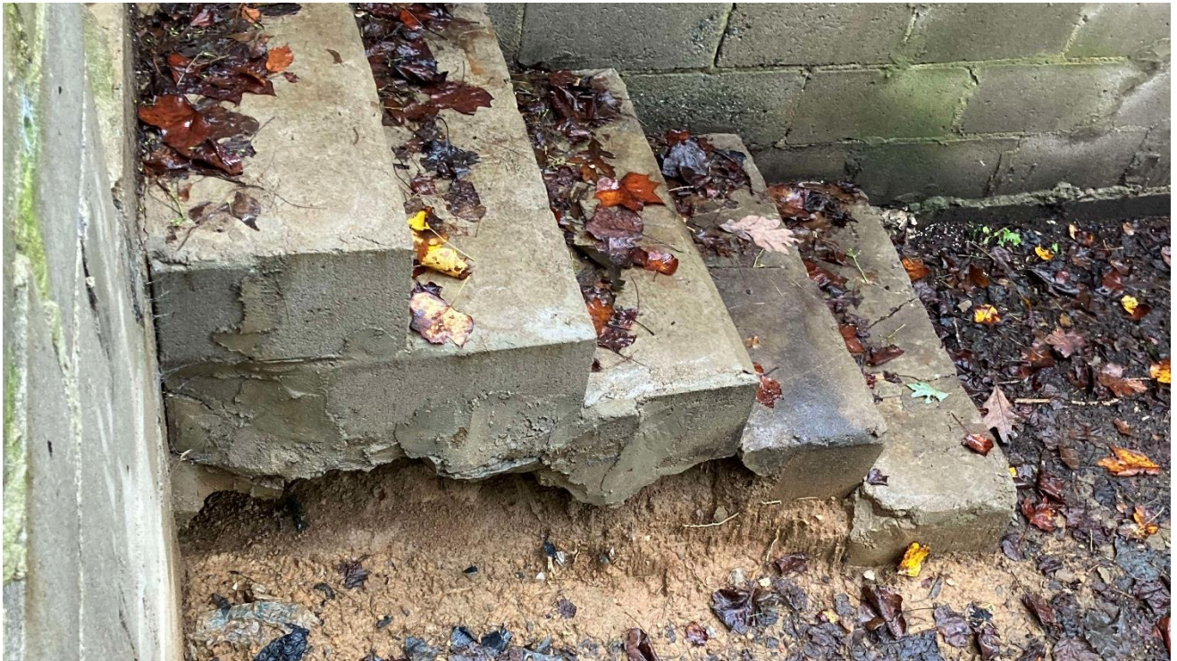
Figure 11 - Erosion Underneath Exterior Concrete Stairs
