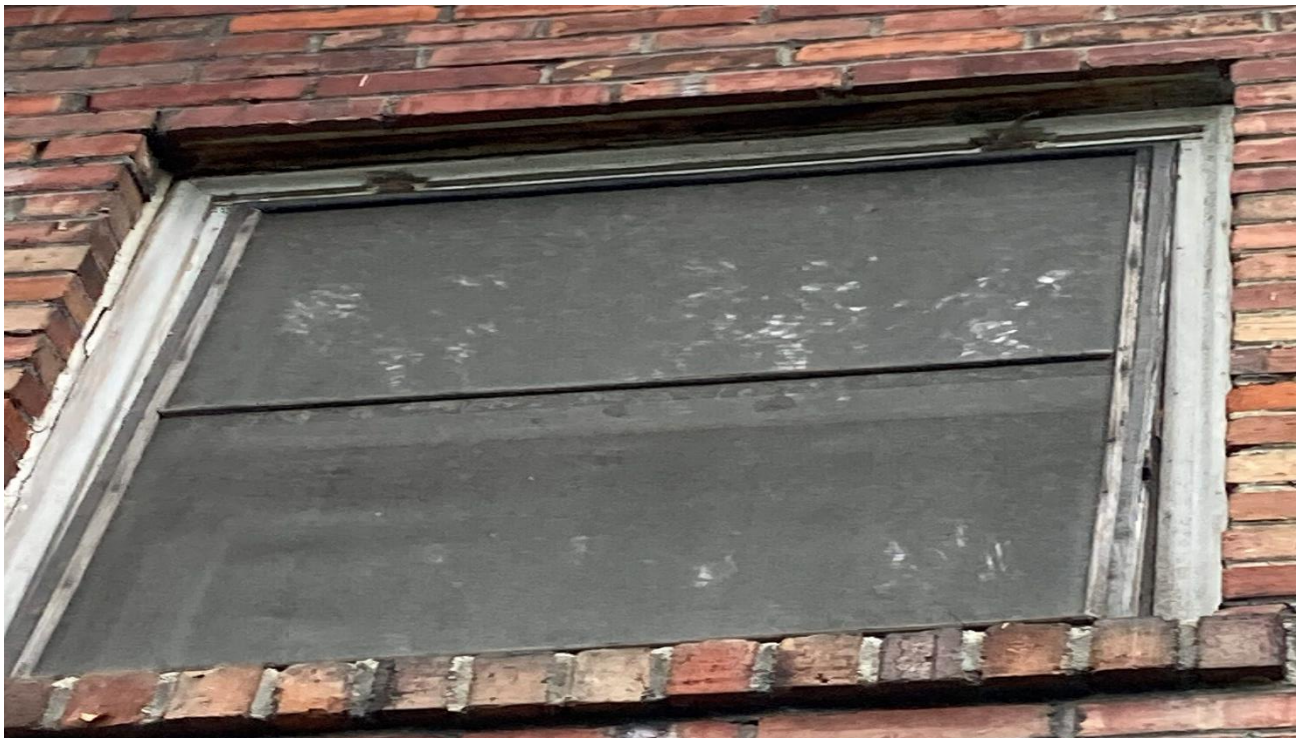
Figure 14 - Rotting Wood Window Frame
