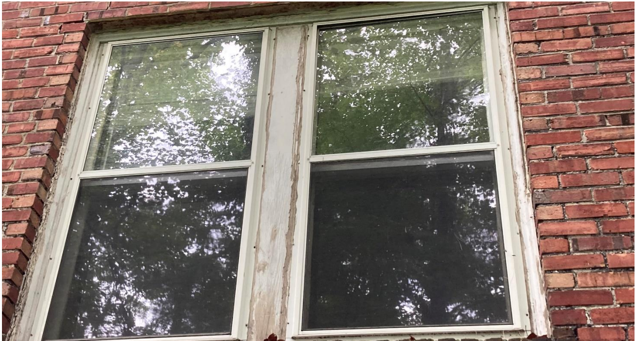
Figure 13 – Rotting/Exposed/Unpainted Wood Window Frame
