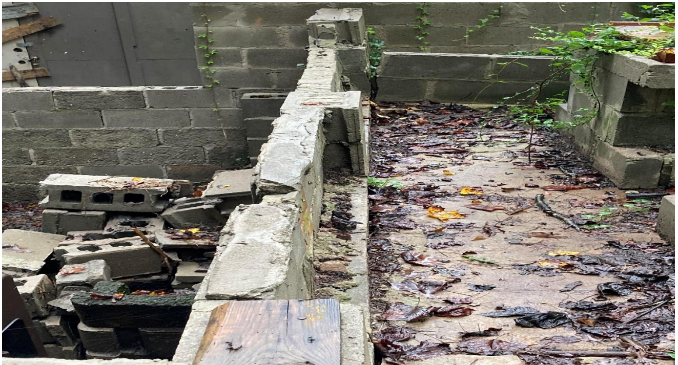
Figure 12 – Leaning Foundation/Wall for Former Boiler Room /Greenhouse
