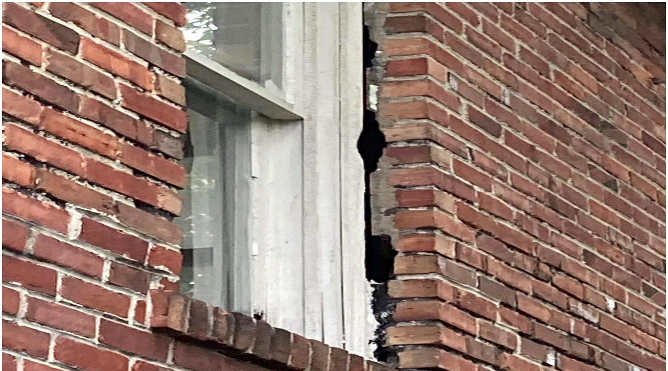
Figure 7 - Gaps between window and frame
