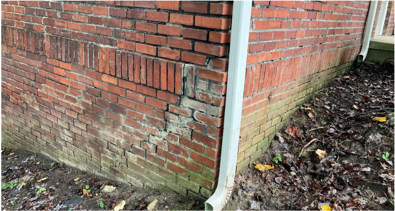
Figure 5 - Cracks in Foundation Masonry
