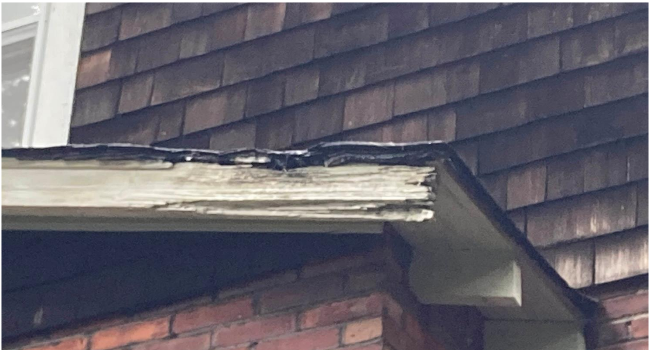
Figure 17 - Damaged/Rotten Eaves and Shingles
