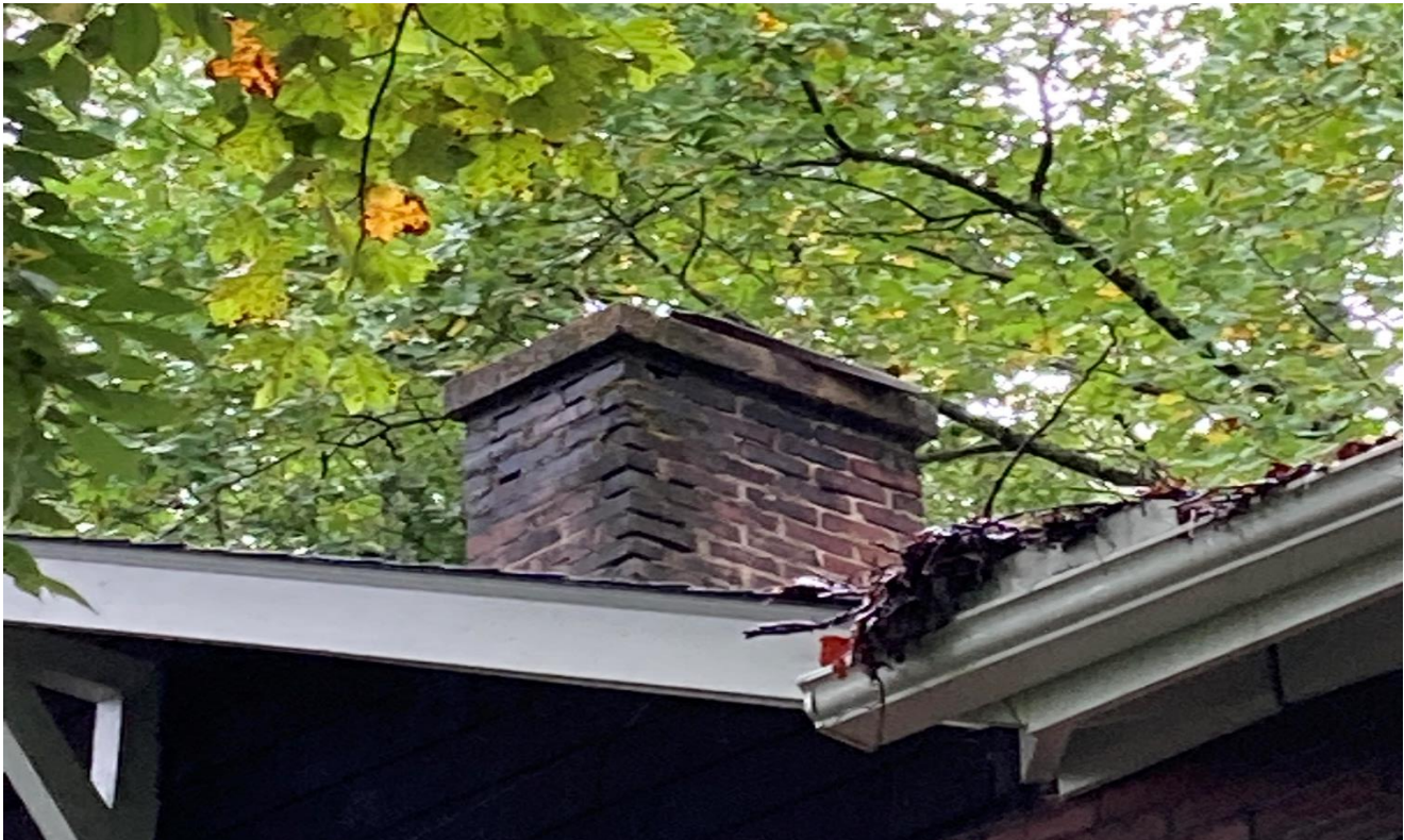
Figure 18 - Missing Mortar on Chimney
