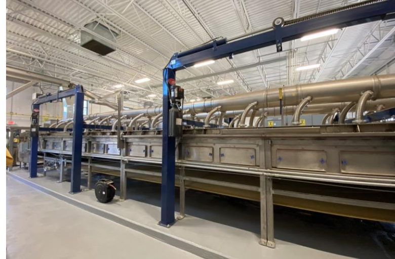
City of Lenoir Lower Creek WWTBiosolids Thermal Drying Facility
