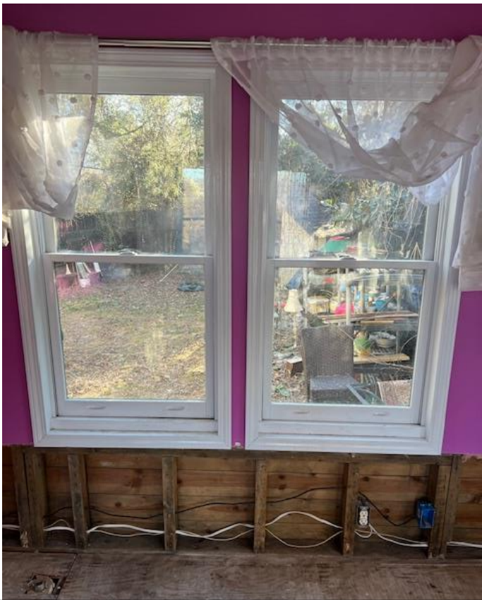
Interior photos of windows proposed to be removed and replaced with double doors.
